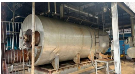
Gambar 3. Unit Boiler PPSDM Migas
