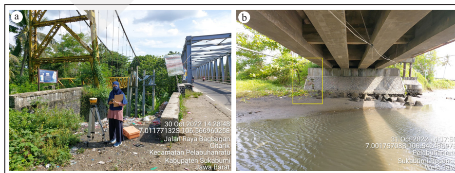
Figure 4. Deformation occurred on huge phase range difference: a) Bagbagan bridge, b) Andira bridge.
